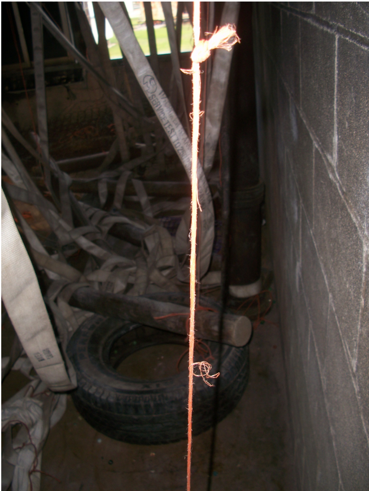
The second-floor obstacles
